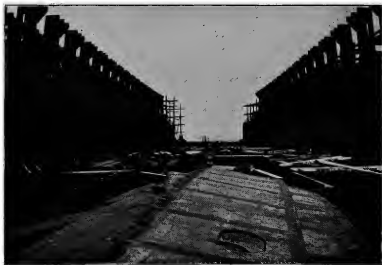
THE HULL OF A STEEL FREIGHTER ABOUT SIXTY DAYS AFTER BEGINNING OF CONSTRUCTION
